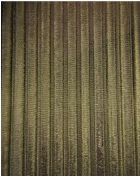
Image of HRSG#51 water preheater tubes with sulfur deposits.
