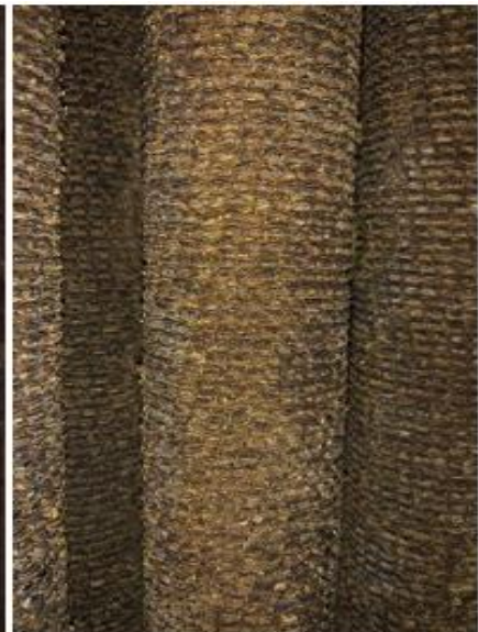
Images of HRSG#51 water preheater tubes with oxidation and corrosion principle.
