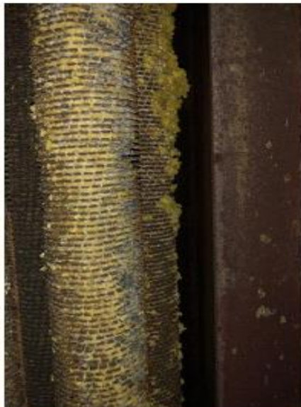
Image of HRSG#52 water preheater tubes with sulfur deposits.
