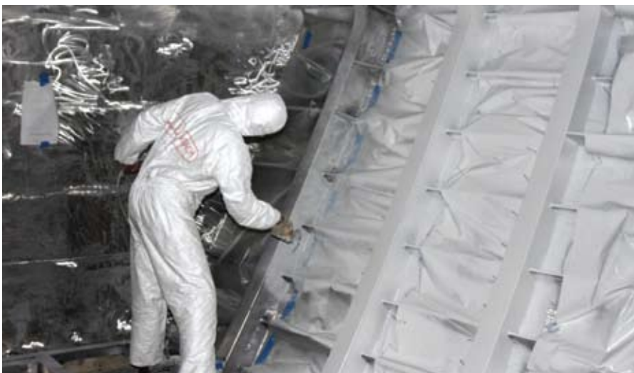
Once traditional insulation gets wet, the material becomes a heat conduit, an odor wick and exposes the metal surface to mold and corrosion. Insulating coatings have no have ability to absorb humidity and cause negative effects, according to Mascoat.
