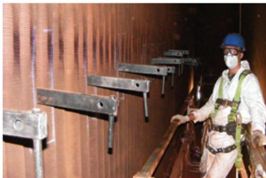
7. Alignment bars are inserted by protected technician to spread tubes and allow deeper penetration of the cleaning wands
