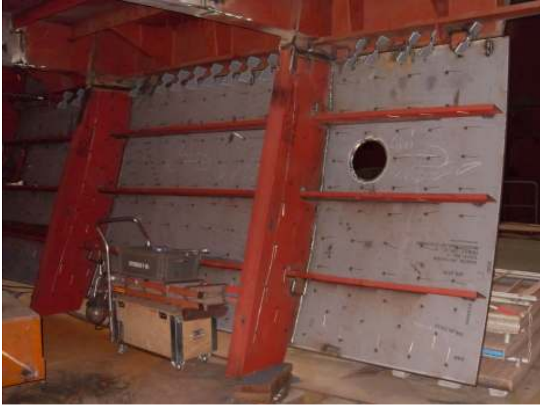
Photo 6: The inner side of the outer shell with needles for fixing the insulation
